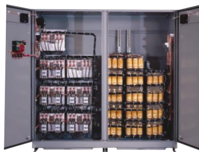
LV Switched Harmonic Filter
