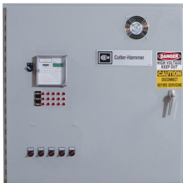
Wall-Mounted Switched Capacitor Bank
